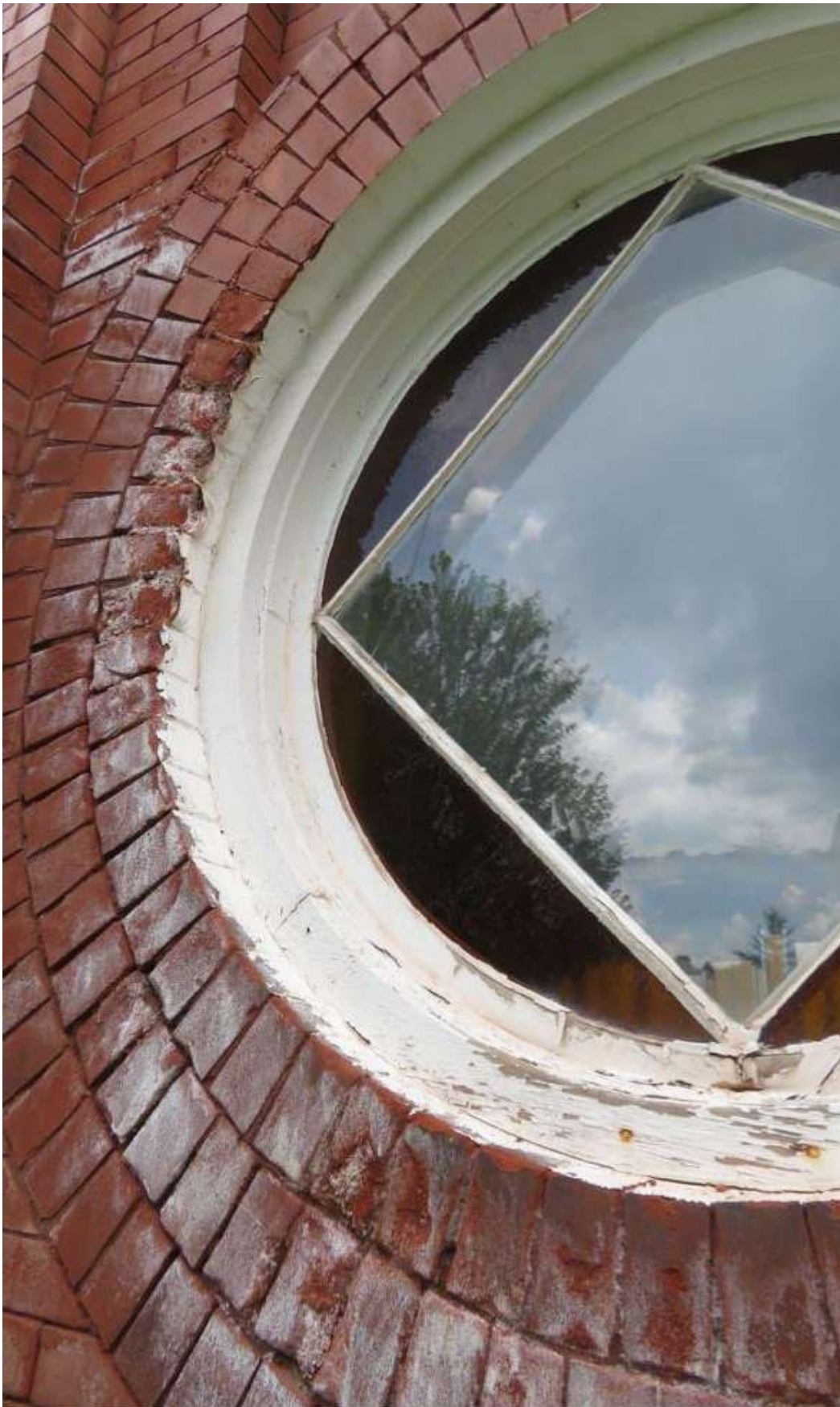
Effloresces, spalled brick, overpainted brick and deteriorated wood
