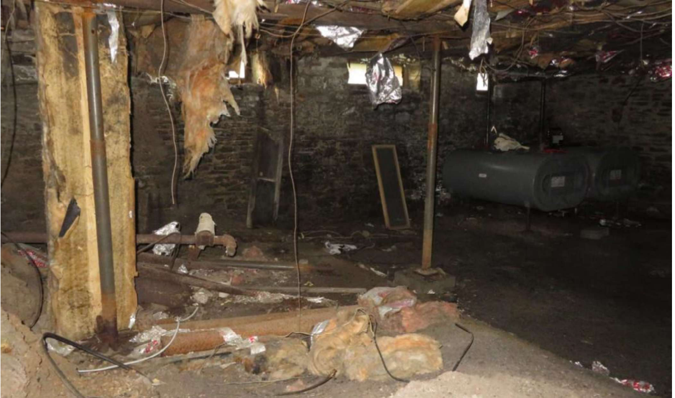
Basement with dirt floor has high moisture levels causing deterioration
