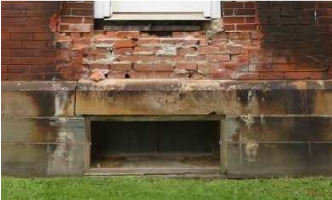
Failing masonry on west wall and basement window
