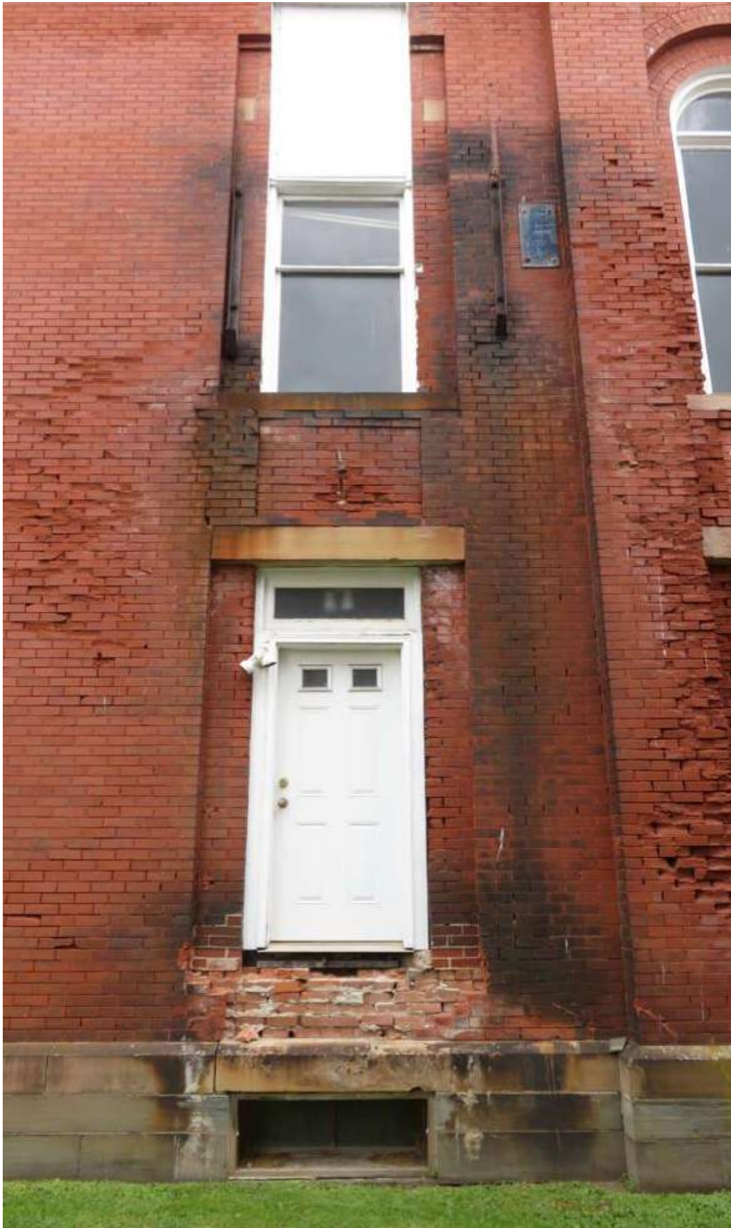
West wall showing severe brick deterioration and altered window openings
