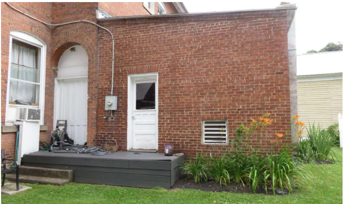
Rear addition showing deteriorated porch and door.
